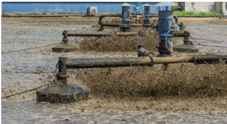
Figure 9: Sludge accumulated in treatment plants can be recycled and used in various fields.
